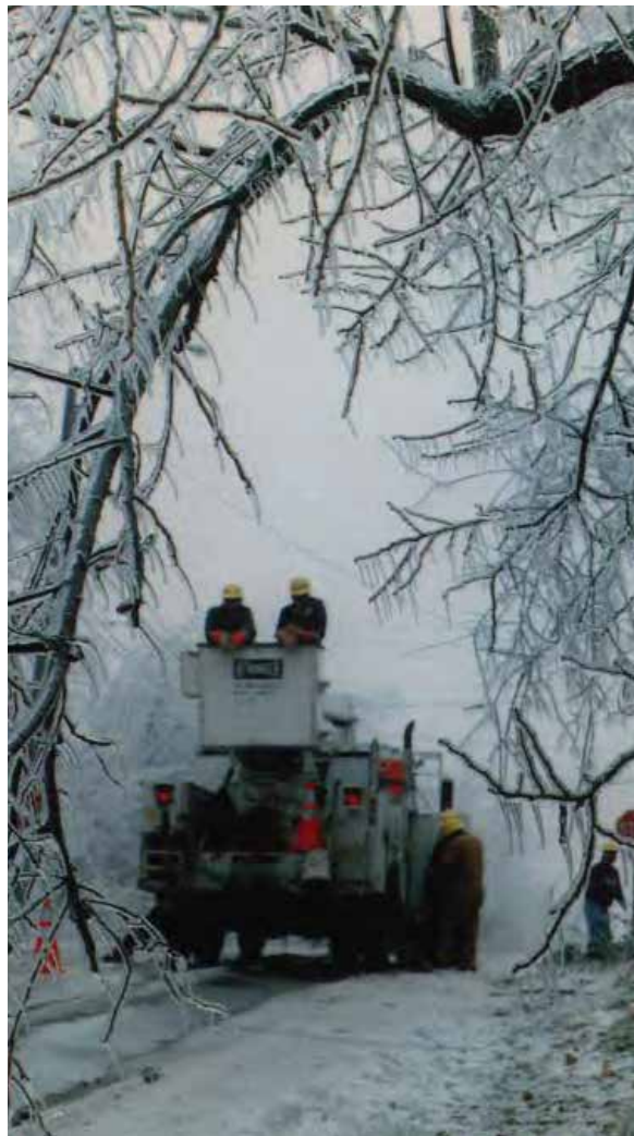
IBEW linemen and utility workers keep the power running during extreme weather
